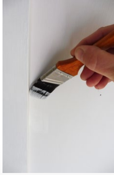
Step six Cut in around the edges of the ceiling and around light fittings with the Resene Ceiling Paint.
