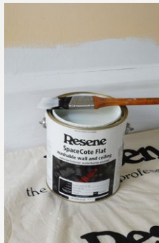
Step ten Cut in around all the woodwork, corners, light switches and sockets with the Resene SpaceCote Flat.
